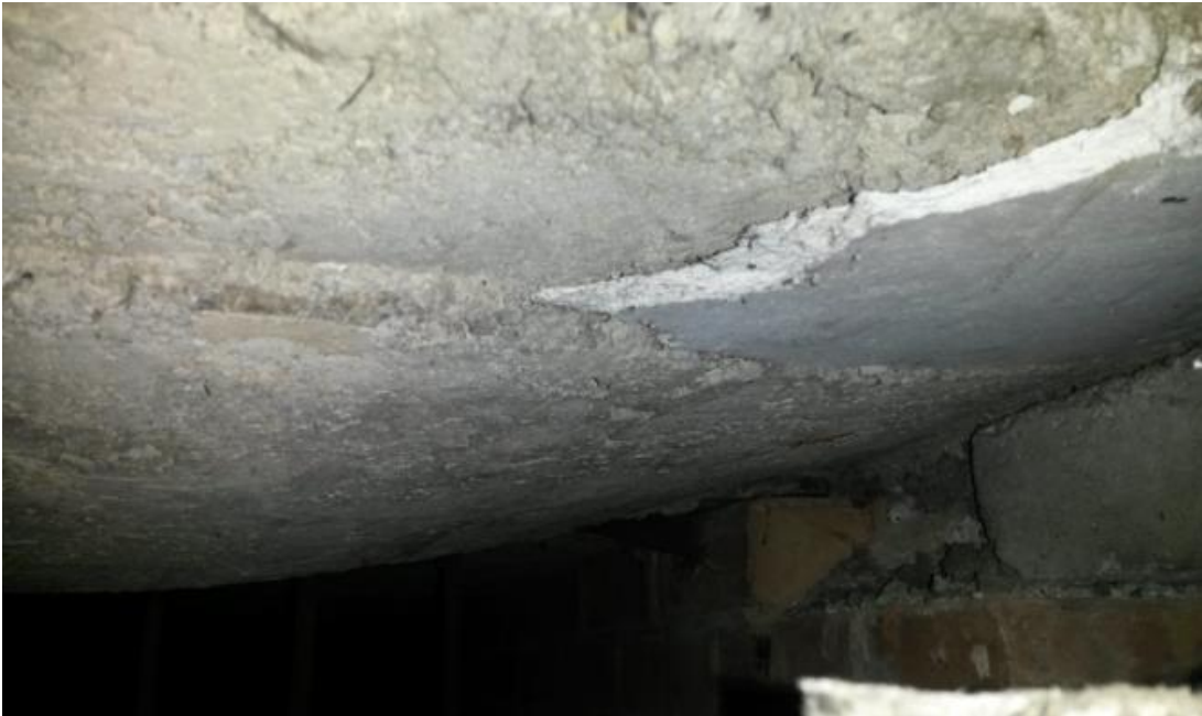
Sub floor heating ducts – insulation board shattering around duct hatches
