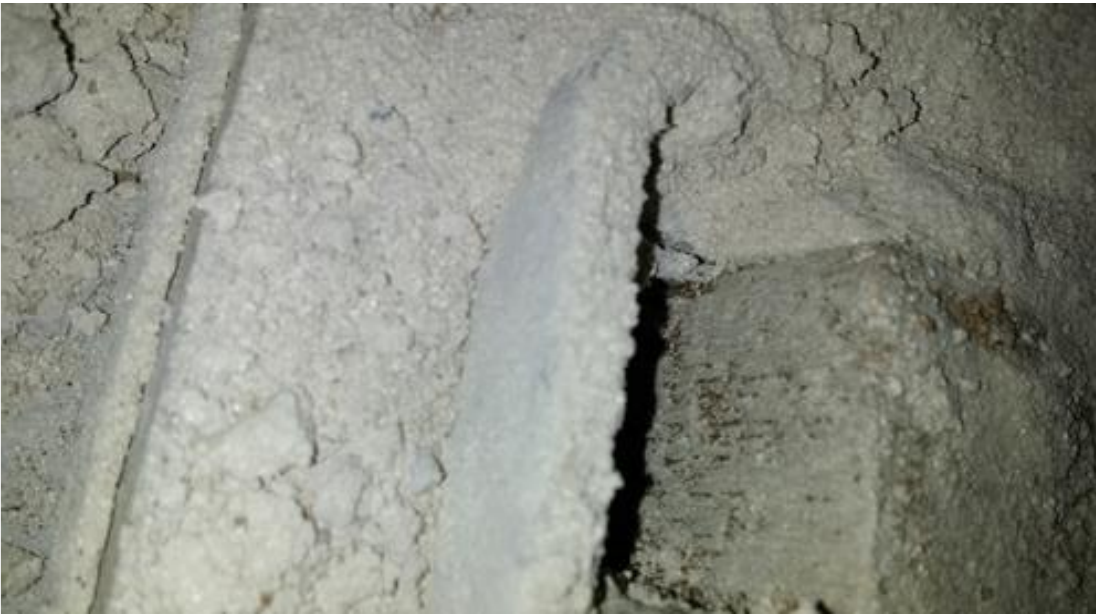
Sprayed asbestos on a column of system built school- CLASP built steel framed school with fully 'lagged' frame
