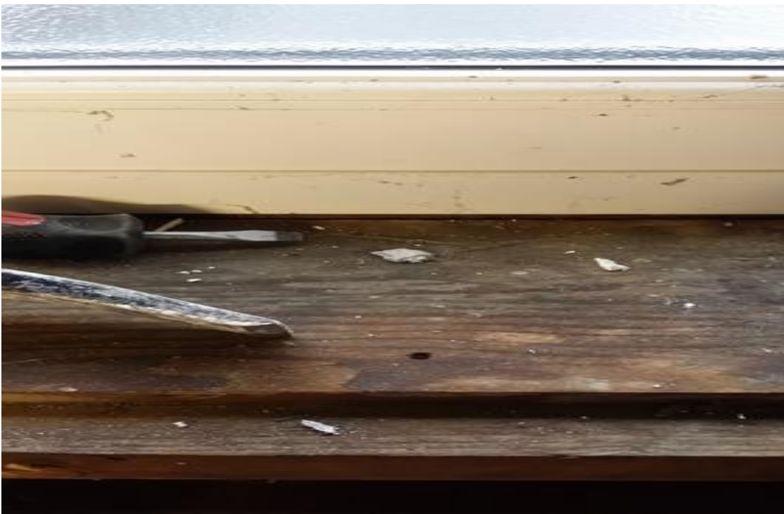
AIB cladding and asbestos debris – asbestos debris from AIB window surround cladding
