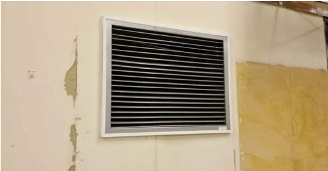
Warm air cabinet heater – AIB Unit 'surround' and internals
