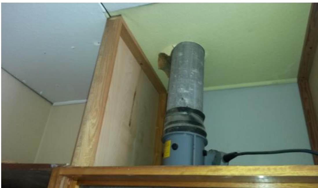
Asbestos cement fume cupboard – cement flue above fume cabinet
