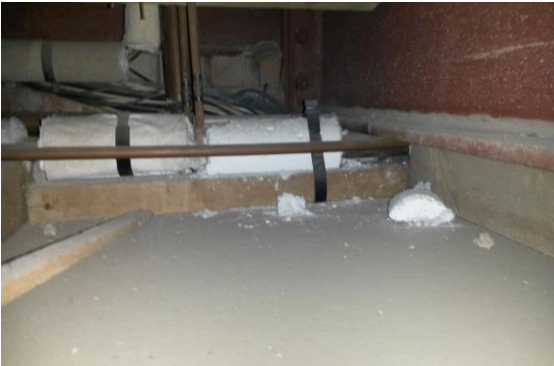
AIB debris in ceiling void of a school - insulation debris to back of non-asbestos suspended ceiling
