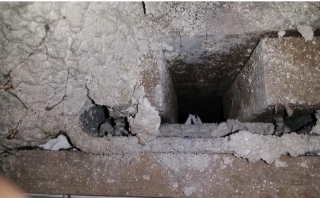
Sprayed asbestos on a column of system built school – lining behind cement wall end and column linings
