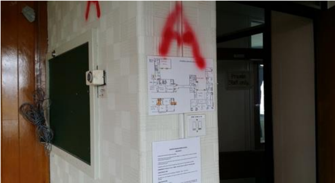
Moulded column cladding containing asbestos
