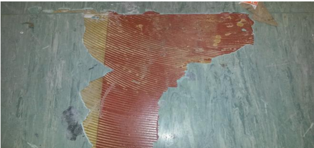
Badly worn asbestos floor tiles in a school corridor – damaged floor tiles and adhesive below corridor carpet
