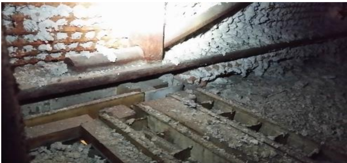
Sprayed asbestos on a column of system built school – Steel frame, wrapped in perforated steel with blown asbestos (note pattern on top left)
